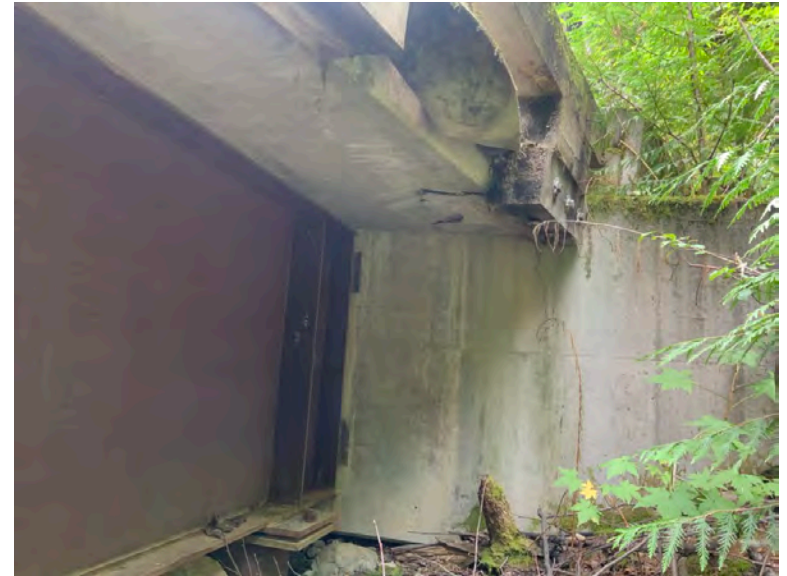
Deck, damage to underside. Right bank u/s
